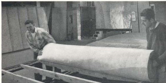
Fast Installation. Two men quickly unroll lightweight Superfine Fiber Glass Insulation on a mobile home roof frame. Easy cutting means correct size every time with little or no wastage.
